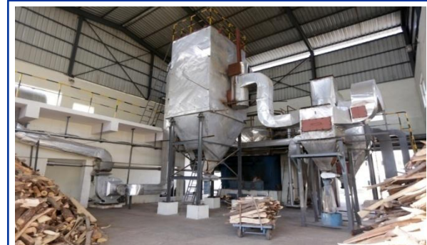
Boiler Equipment View
