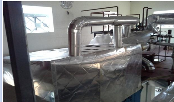
Boiler Equipment View
