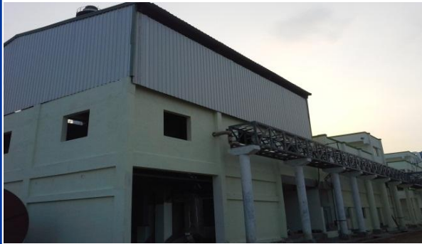
Boiler House Overview
